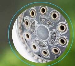
Mineral buildup on fixtures & components
